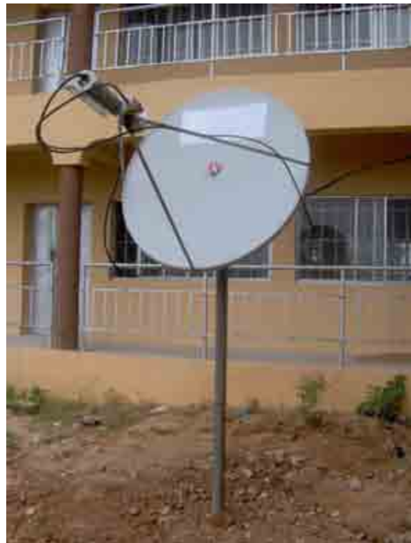
Plate1: Location of the Very Small Aperture Terminal (VSAT).
